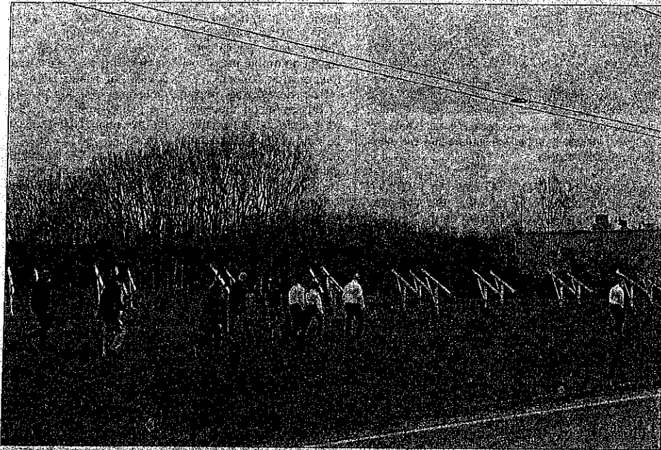
After a press conference on April 20, Bendix managers and employees toured the site where the 2,612-panel solar array will soon stand. Construction on the project began this month and is scheduled to be completed in September.
